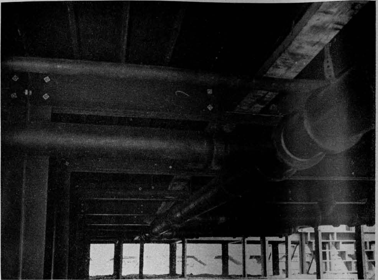
Figure 39. View under floor showing piping.
