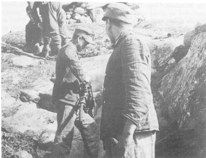
Engineer using jackhammer to break up rocks for the construction of positions on the Litsa River front.
